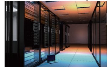
Data center thermal management
